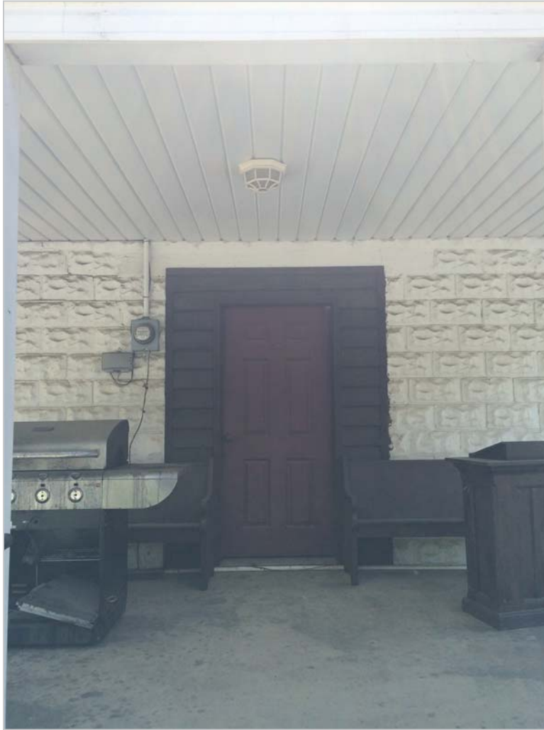
Photograph 3: Replacement door of the original church on the north facade; looking south.
